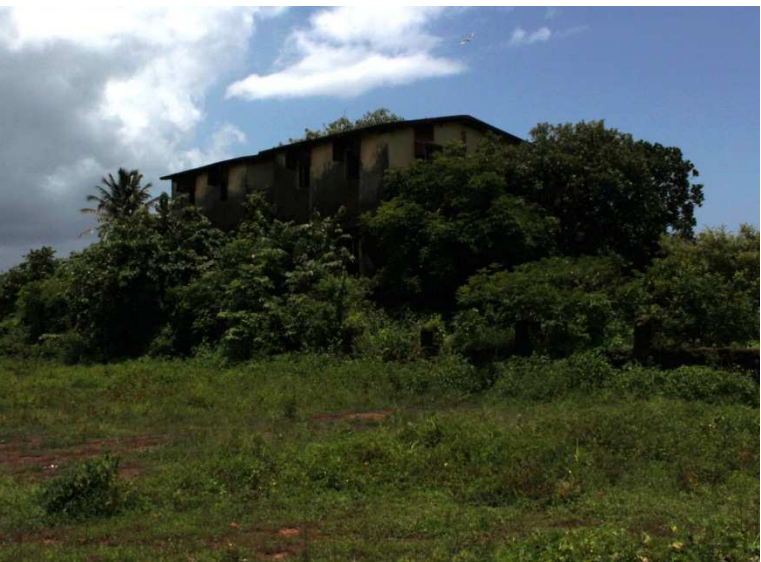
Existing dilapidated structure of MMTC staff quarters 7
